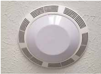
Lighted Bathroom Vent
